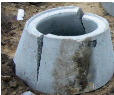
Photo 6: Broken concrete cone
