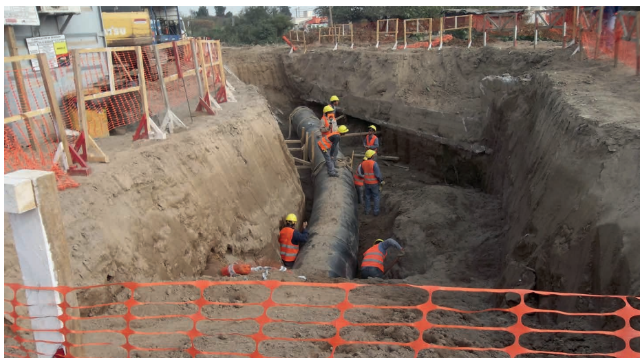
Photo 2: Long-term conditions, of a bended Krah Pipe DN/ID 1300 mm
