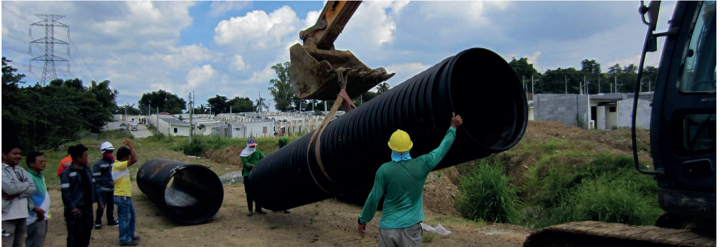
Photo 3: Lifting of 6 meters length, 1000mm krah profiled wall pipe assisted by site workers on site
