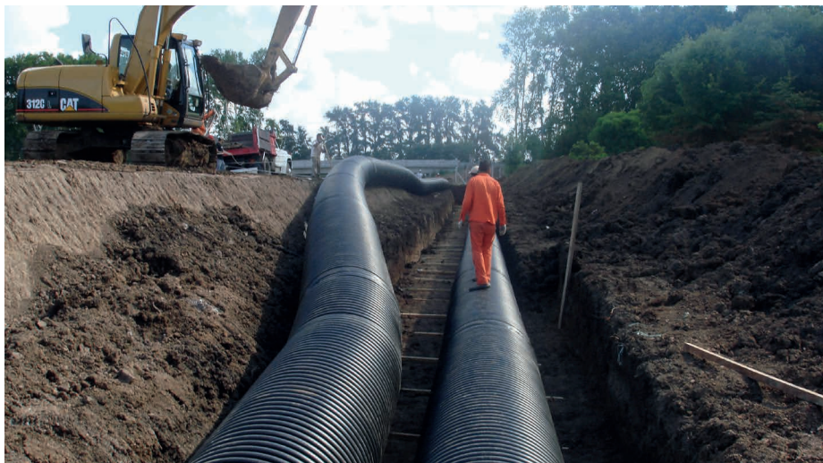
Photo 1: Short-term bending conditions, the welding was done outside and now the pipe is moved into the trench DN/ID 1200 mm
