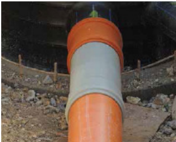
Figure 10: HDPE to uPVC, including "Rocker Section"
