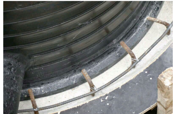
Figure 8: Krah HDPE Manhole positioned on top of precast base slab (note steel ring for “Upturn Beam”)
