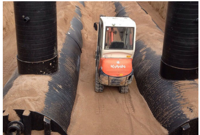
Pic. 7: Double wall Leachate-reservoir (Henze GmbH, RBV Pöthe, Germany)
