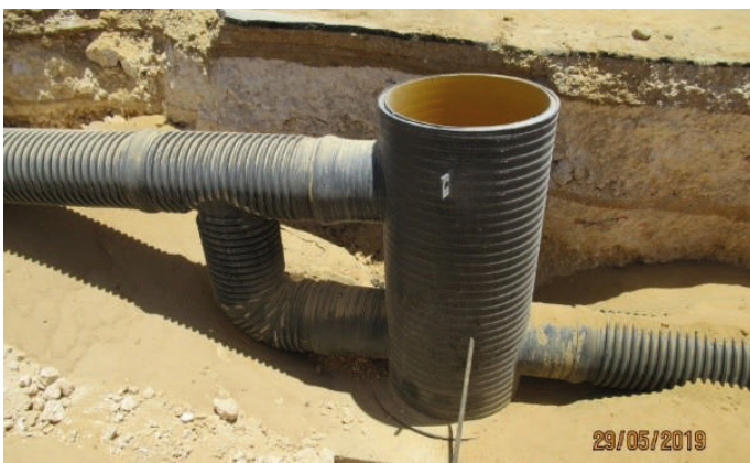
Manhole with external backdrop
