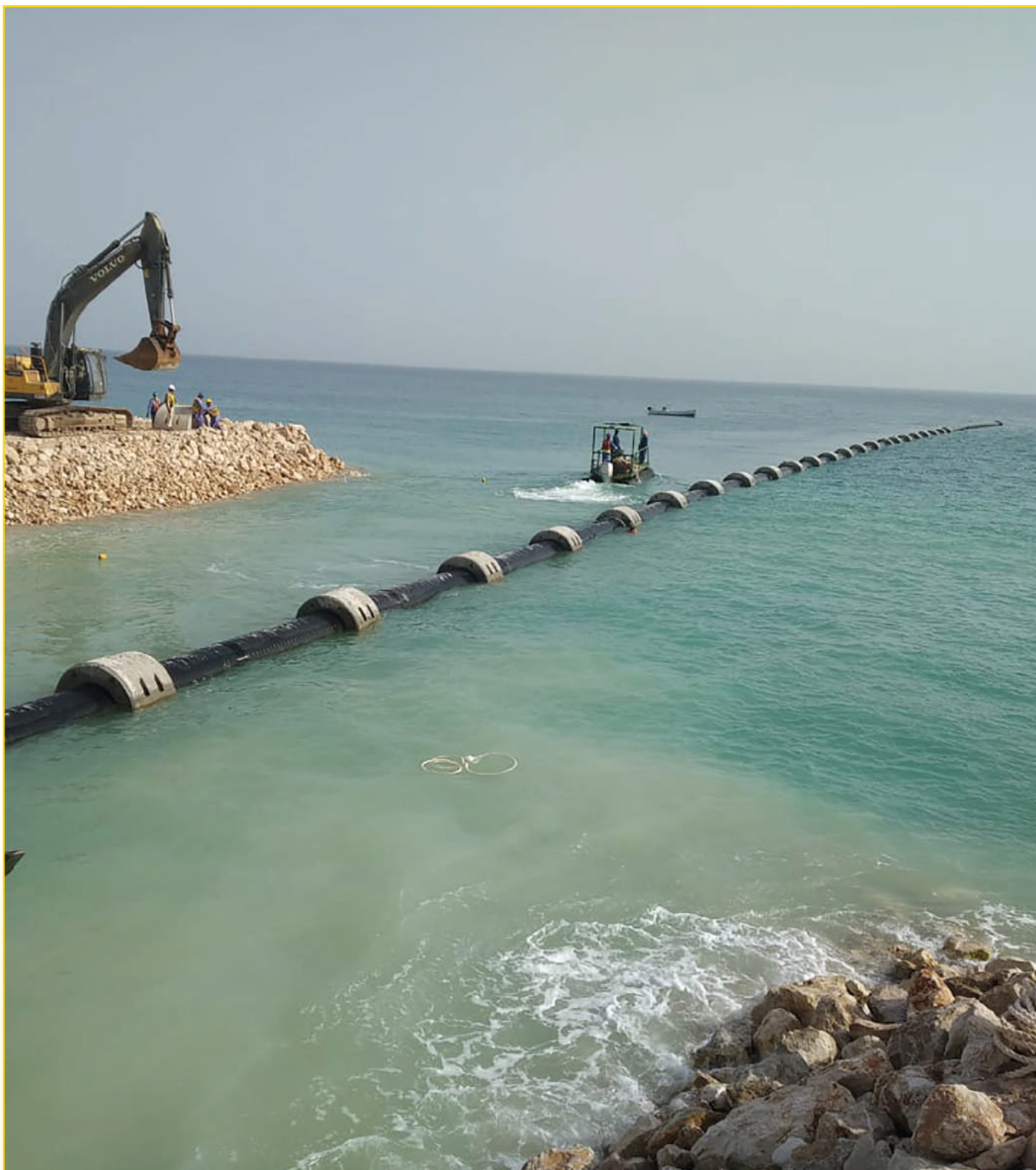
Overview of the big installation site in Salah
