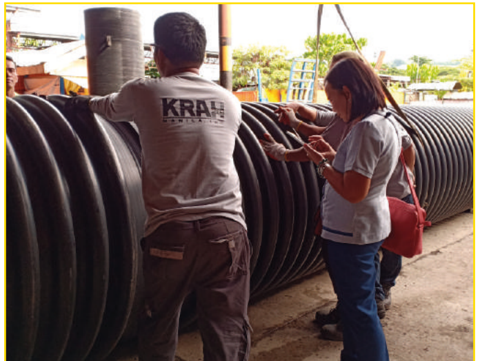
Electrofusion jointing off-trench of DN/ID 1800 mm along Brgy. Balagbag in Boracay Island
