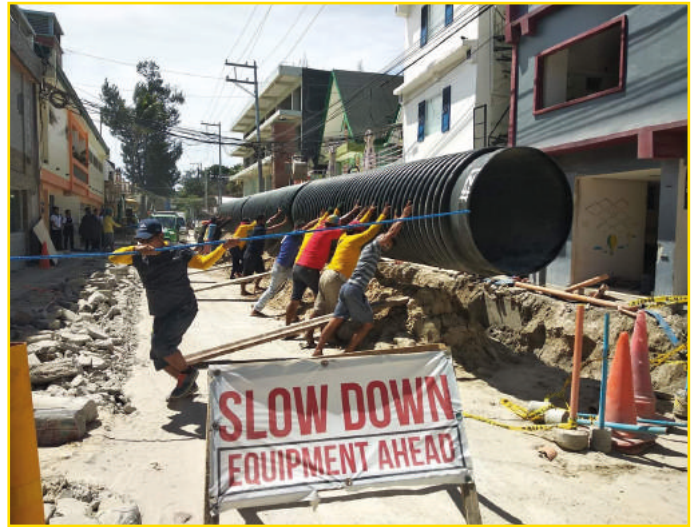
No heavy machinery is needed, pure manpower can install a Krah pipeline!
