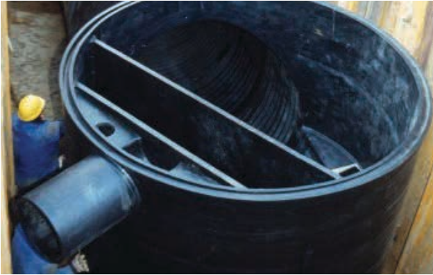
Storm water retention tank
