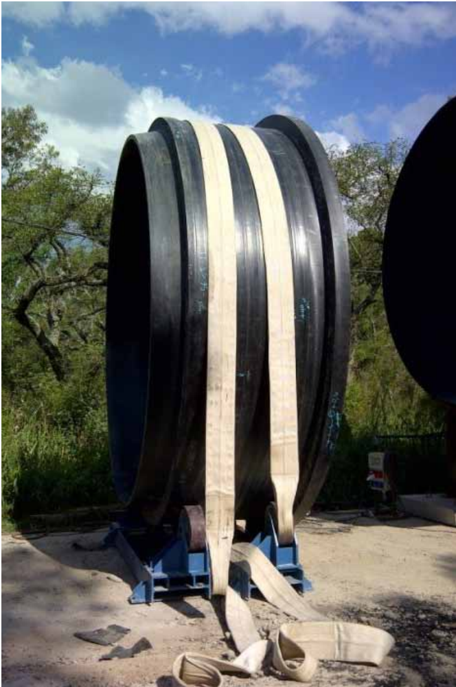
Flange connection between the two pipe ends
