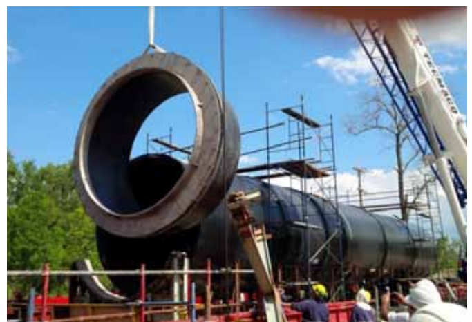
Flange connection between pipe and concrete basin
