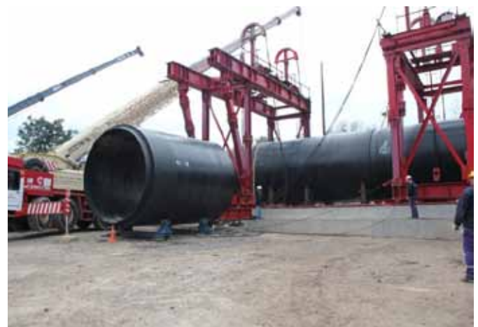
Process- and treatment station on site
