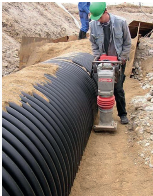
Pic 4: Krah Pipes Oman
