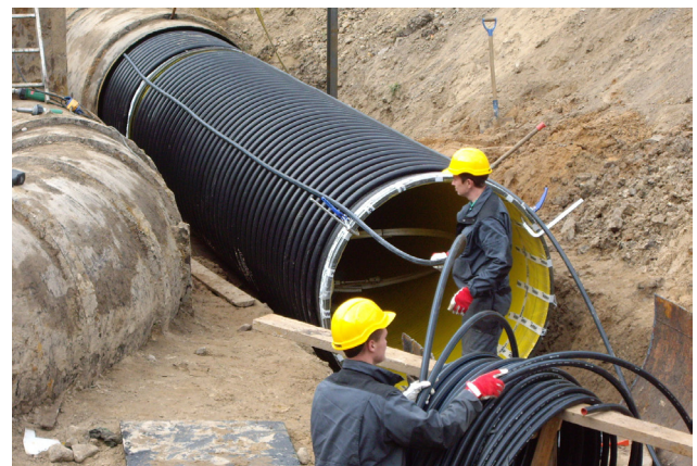
Start point of the relining, Krah electro-fusion welding and bentonite pipe installation
