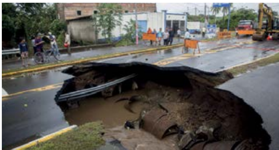
Pic. 3: The failure here was a broken drainage pipe. Source: ABCNews
