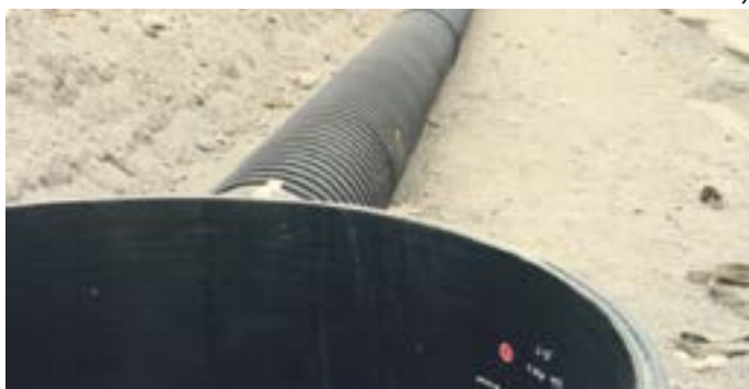
Picture 3: Free installed Krah sewer pipe DN/ID 1000 mm with profiled wall for anchorage
