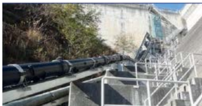
Picture 2: Krah pressure pipe with clamps and concrete fix points for hydropower plant
