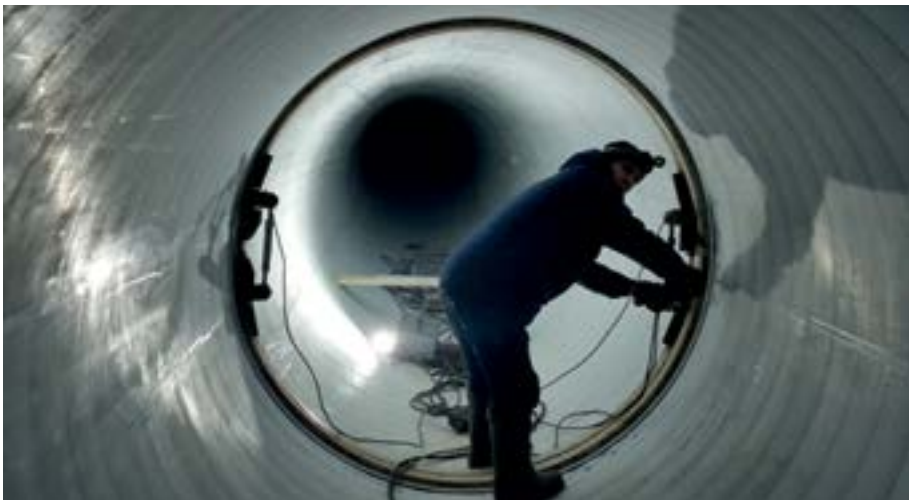
Pic. 2: Welding of CORSYS PLUS DN/ID 2000 mm from inside using two welding units. The pipes are already installed in the renovated conduits.
