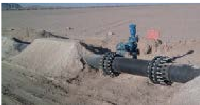
Picture 1: Free installed Krah pressure pipe (PE-GF) with partially embankment for mine industry
