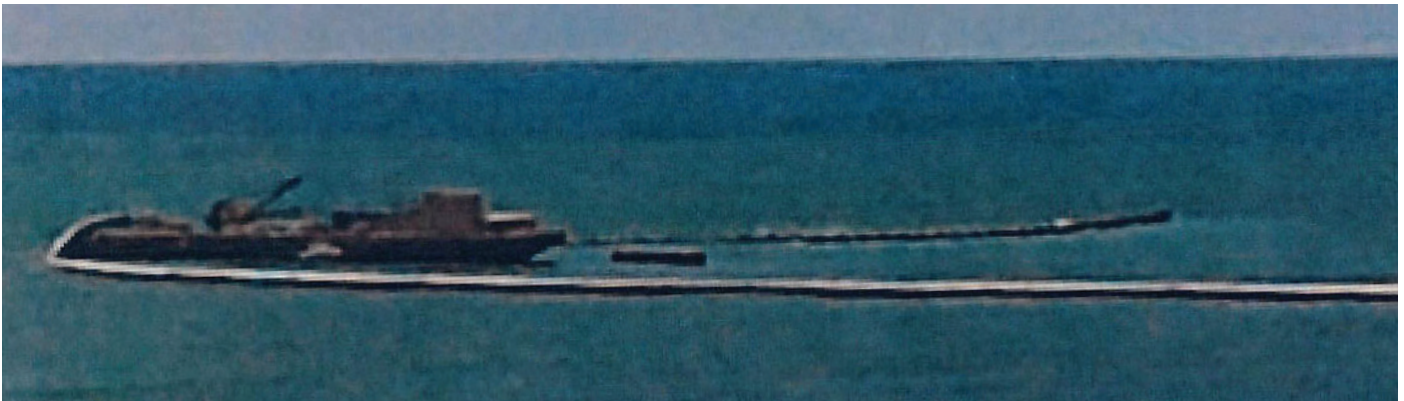
During installation of an outfall pipeline supplied from north of Europe to Latin America, a pipe has broken.
