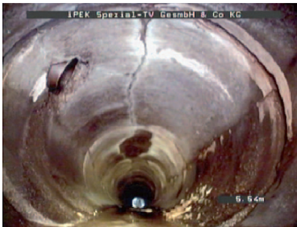
old and damaged sewer
