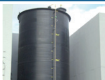
Storage tanks and special apparatus
