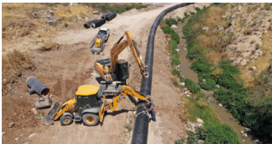
Temporary pipeline along Kidron Wadi
