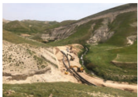
Eastern pipelines section
