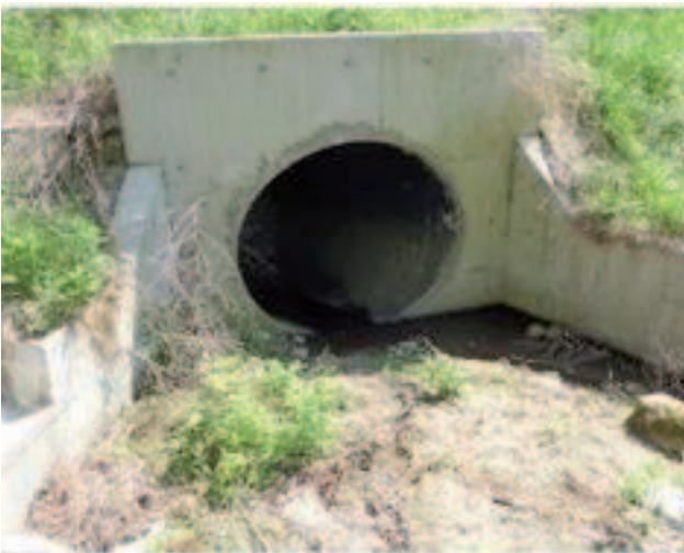
Rikuzen-takata city ,Iwate Pref. 1000mmID , Total length are 80m. We didn't have any damage of appearance with naked eyes. Maximum deflections are 4.2% in upstream area
