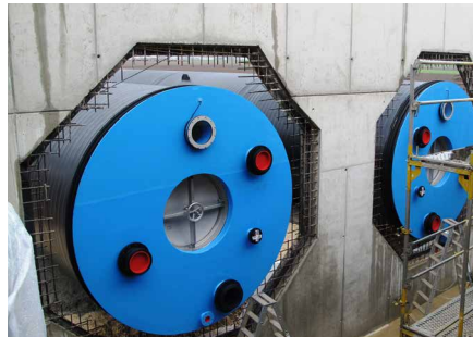
Pic 5 : Integration of the two functional walls in the outer wall of the waterworks
