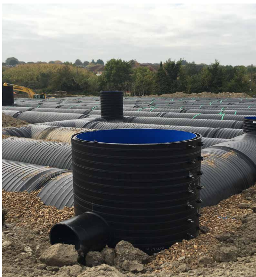
Pipeline with inspection chamber
