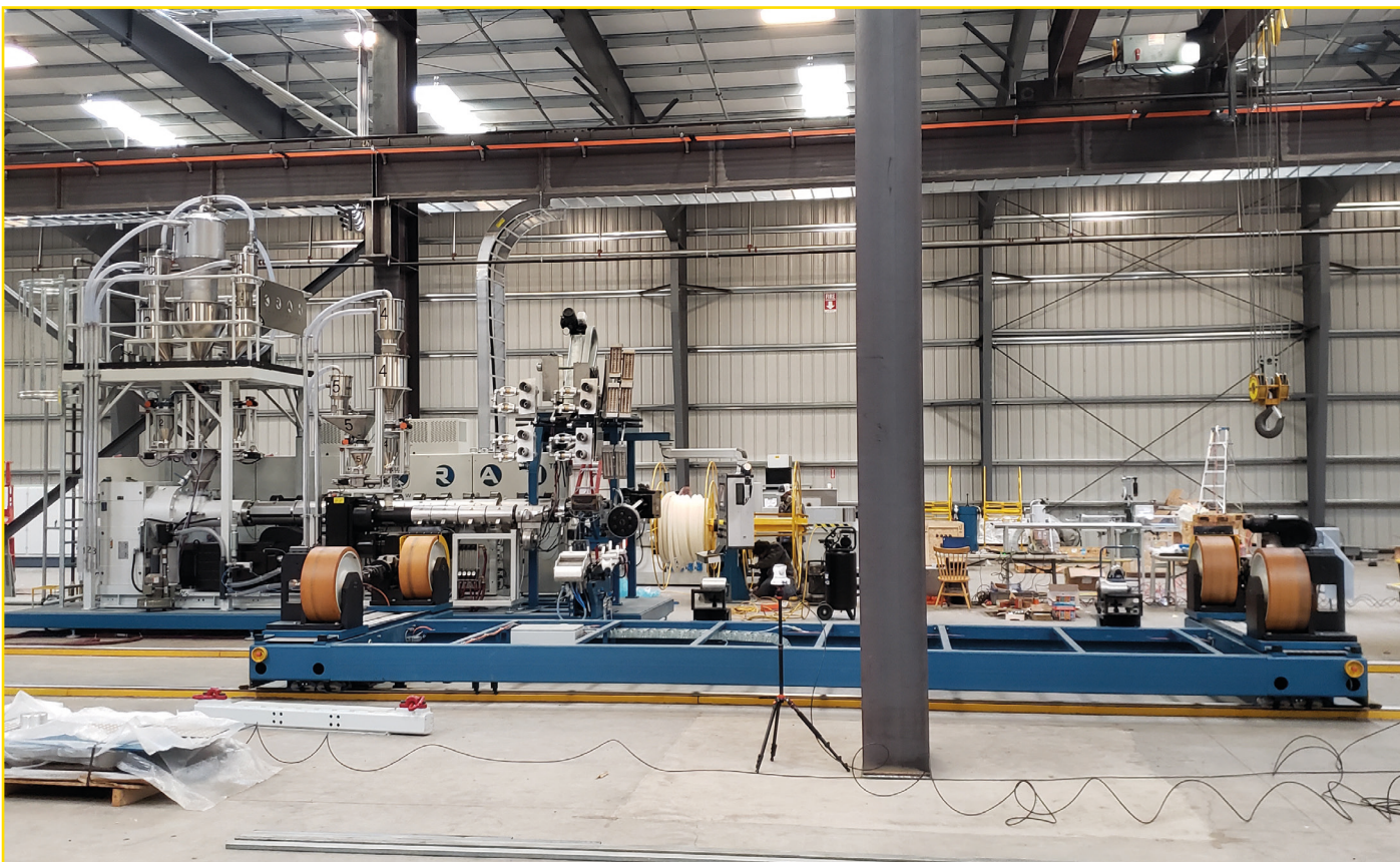
The new machine during installation, next to the grey pillar you can see one of the virtual assembly cameras
