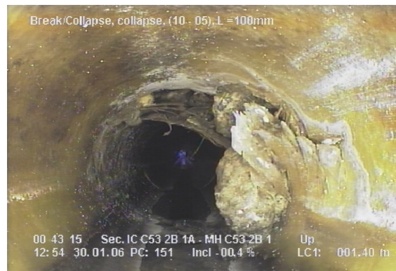
Complete pipe break of GRP pipe.
