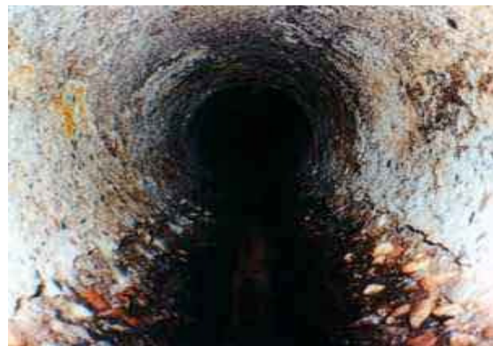
Internal corrosion in a concrete pipe
