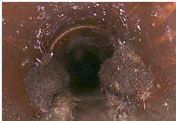
Growing roots after cracking
