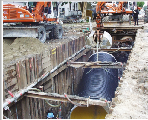
Sewer pipeline DN/ID 2000mm (79")
