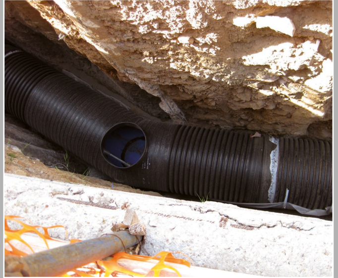
Storm drainage line with integrated manhole
