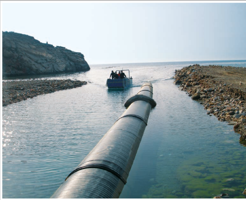
Outfall pipe line DN/ID 2000mm (79")
