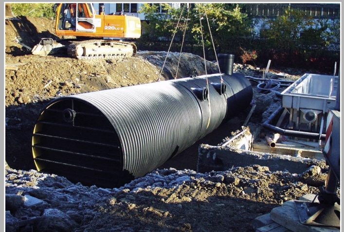
Retention tank of a public swimming pool, DN/ID 3000mm (118")
