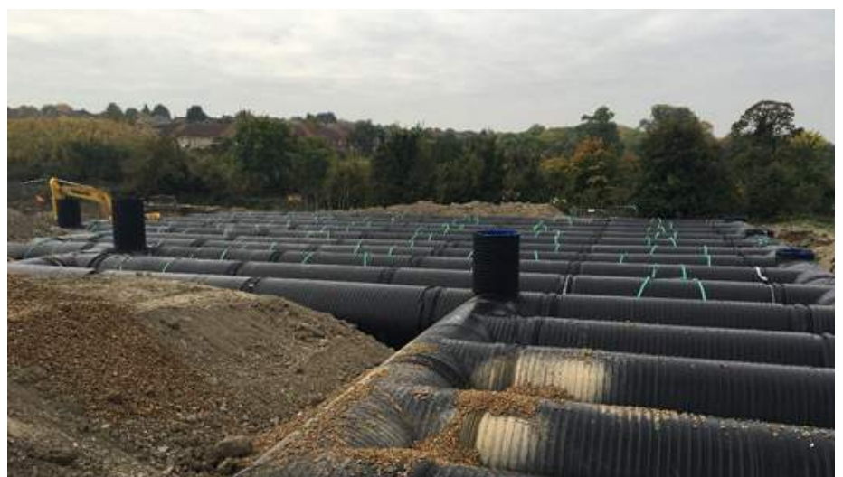
Figure 4. Large diameter pipe stormwater attenuation structure on a residential development in the UK
