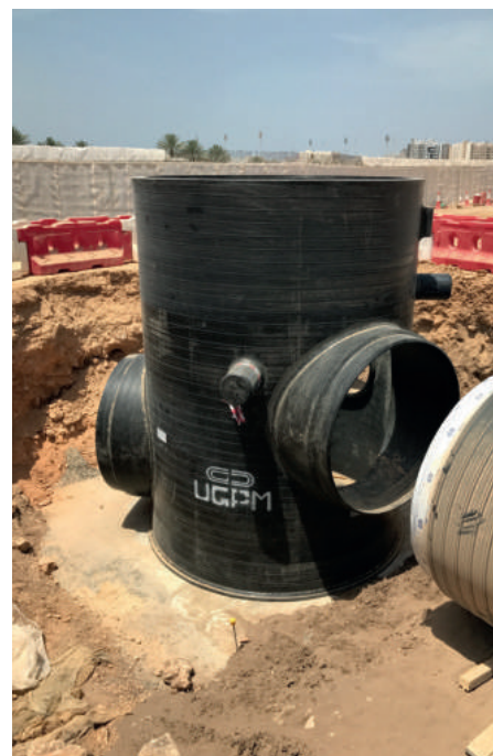
Stormwater system for Mall of Oman, produced by UGPM
