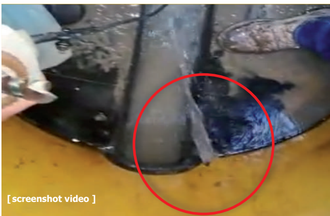
Heavy infiltration of water in the manhole
