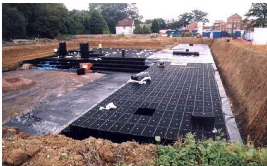
Figure 5. A geocellular stormwater attenuation structure on a residential development in the UK
