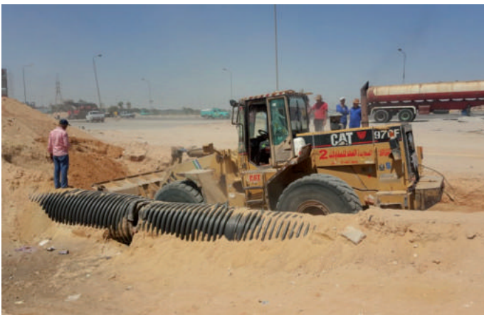
The broken pipe
