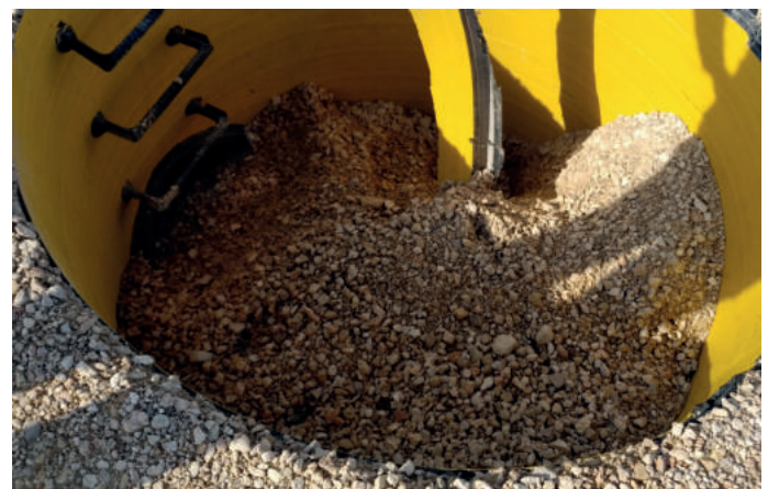
A manhole filled by gravel, due to leakage
